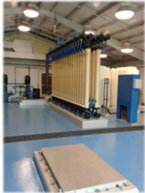
Horn Creek Microfiltration System
